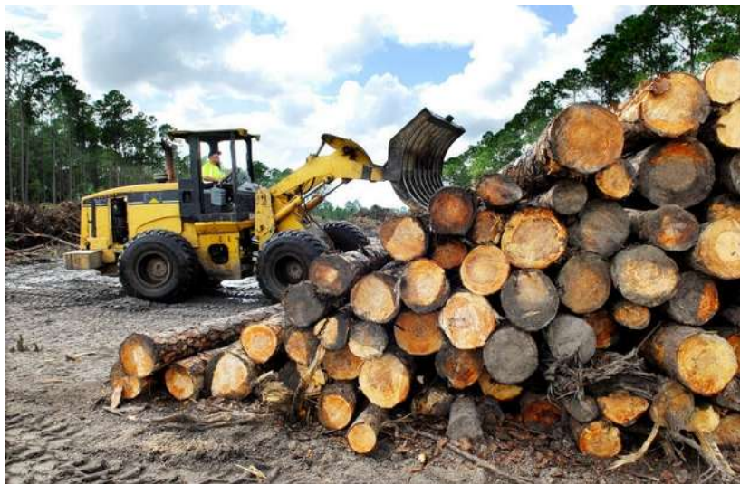
David Oliver of Ft. Pierce drives heavy equipment to clear woods for the Palm Bay Parkway. Construction is scheduled to take about 18 months, with the new road expected to be ready by spring 2014.
